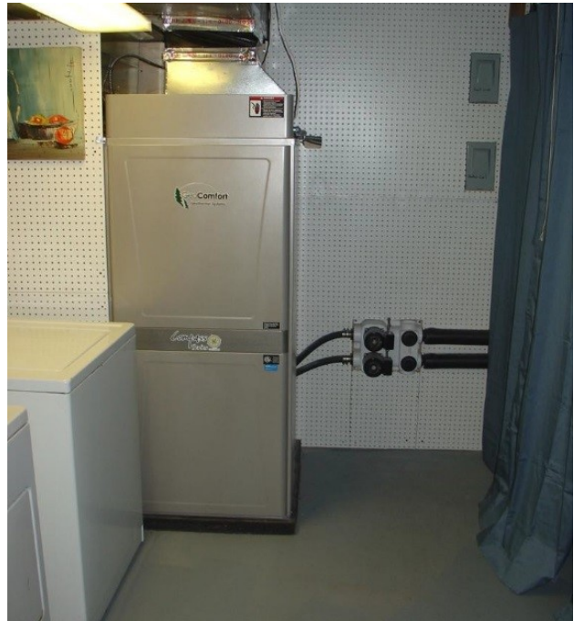
Ground Source Geothermal Heat Pump Furnace Replaces Unsustainable Natural Gas Burning Furnace
