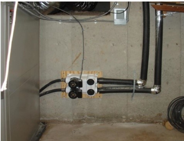
Ground Loop in the basement with two circulation motors
