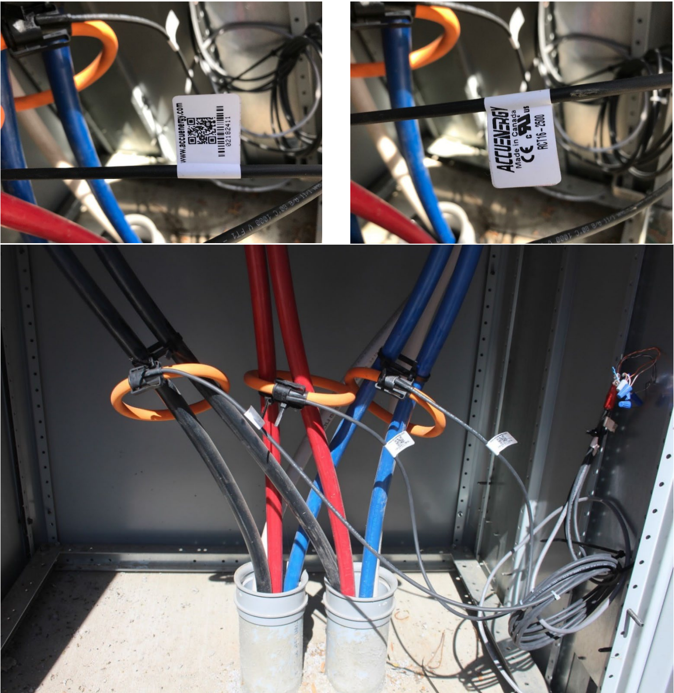
Figure 88 Rope CTs used to monitor the current in the main lines to the facility appear to be properly installed.
