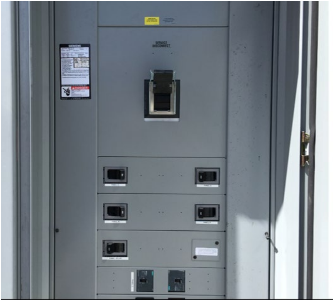
Figure 93 Main Distribution Panel
