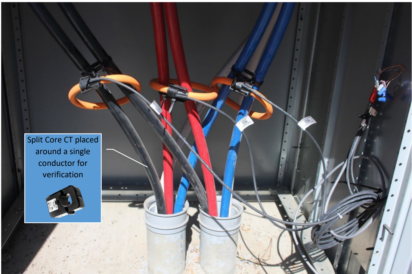
Figure 90 Split Core CTs were also added to individual conductors to verify the output of the Rope CTs
